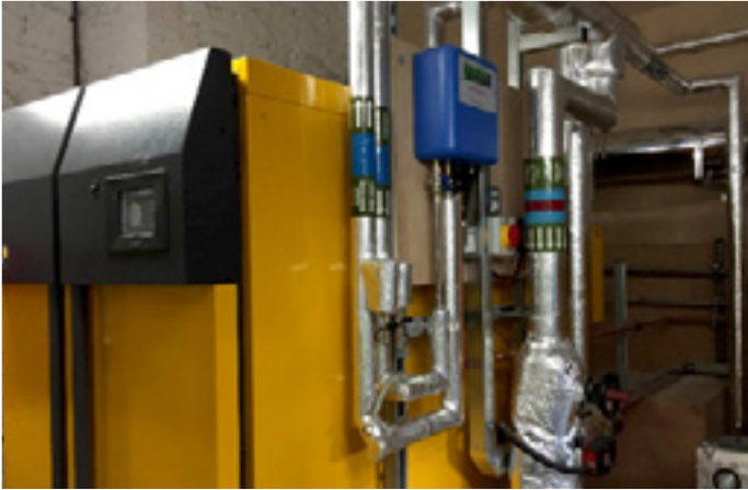
↑ 220kW pellet boiler at Saltram House
