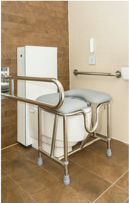
↑ WALL-MOUNTED GRAB RAILS FOR ADDITIONAL SUPPORT
